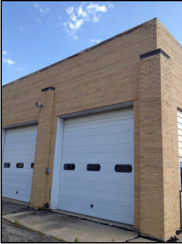
Photo #11: North Elevation – overhead door conditions.
