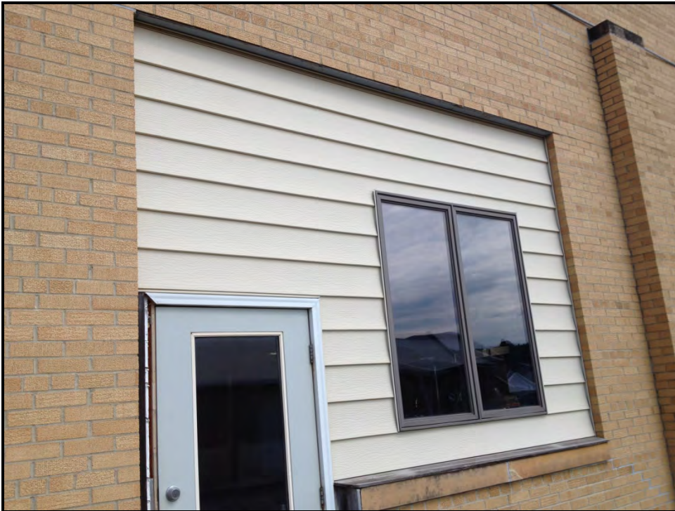
Photo #12: West Elevation – siding, door and window condition.
