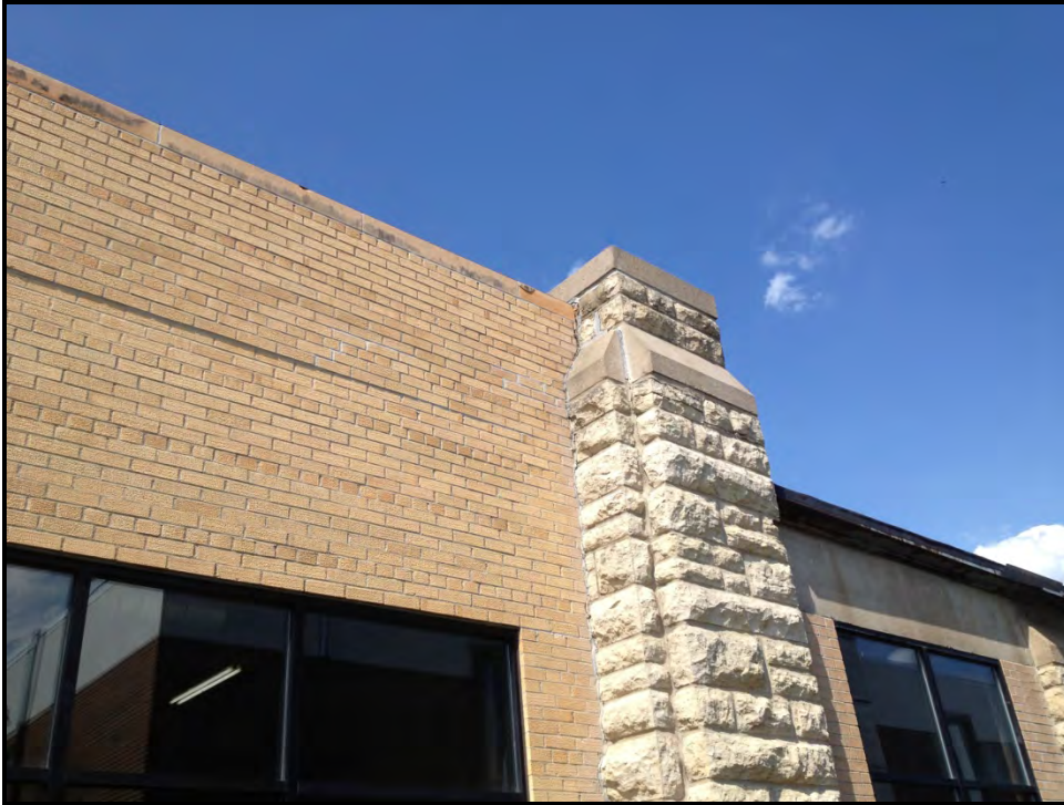
Photo #15: South Elevation – limestone condition.
