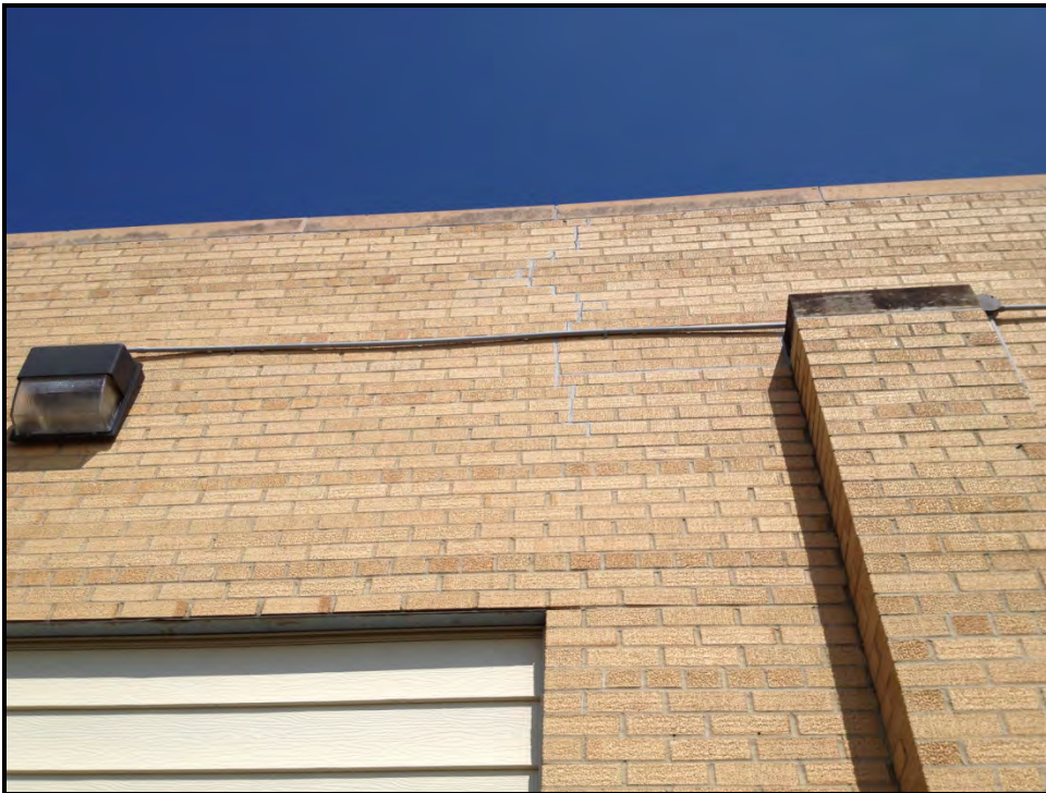
Photo #20: West Elevation – stress crack in brick veneer.
