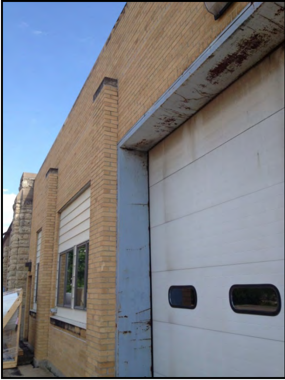
Photo #9: North Elevation – overhead door conditions.
