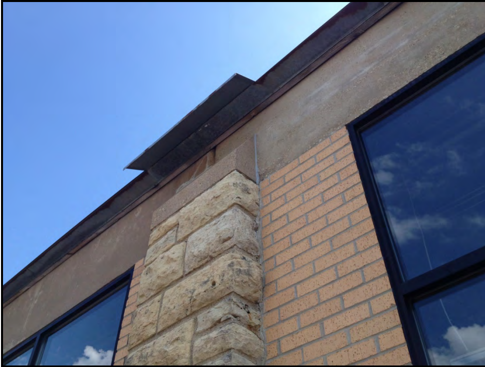
Photo #3: North and South Elevations – roof condition at limestone pilaster.
