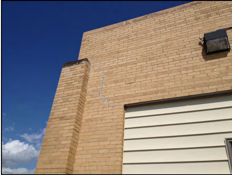
Photo #1: West Elevation – stress crack in brick veneer.
