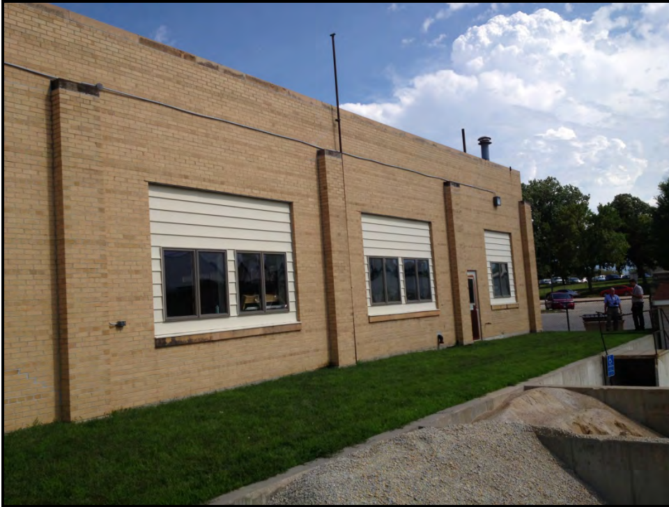
Photo #13: West Elevation – brick veneer condition. Needs safety barrier.
