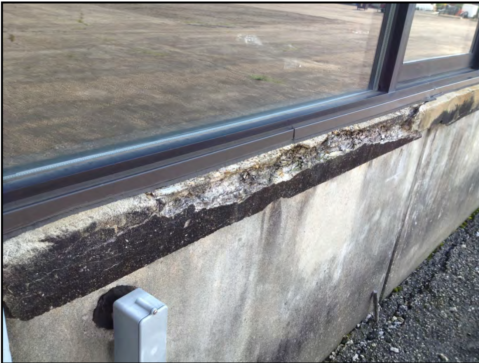
Photo #20: Typical window sill condition.
