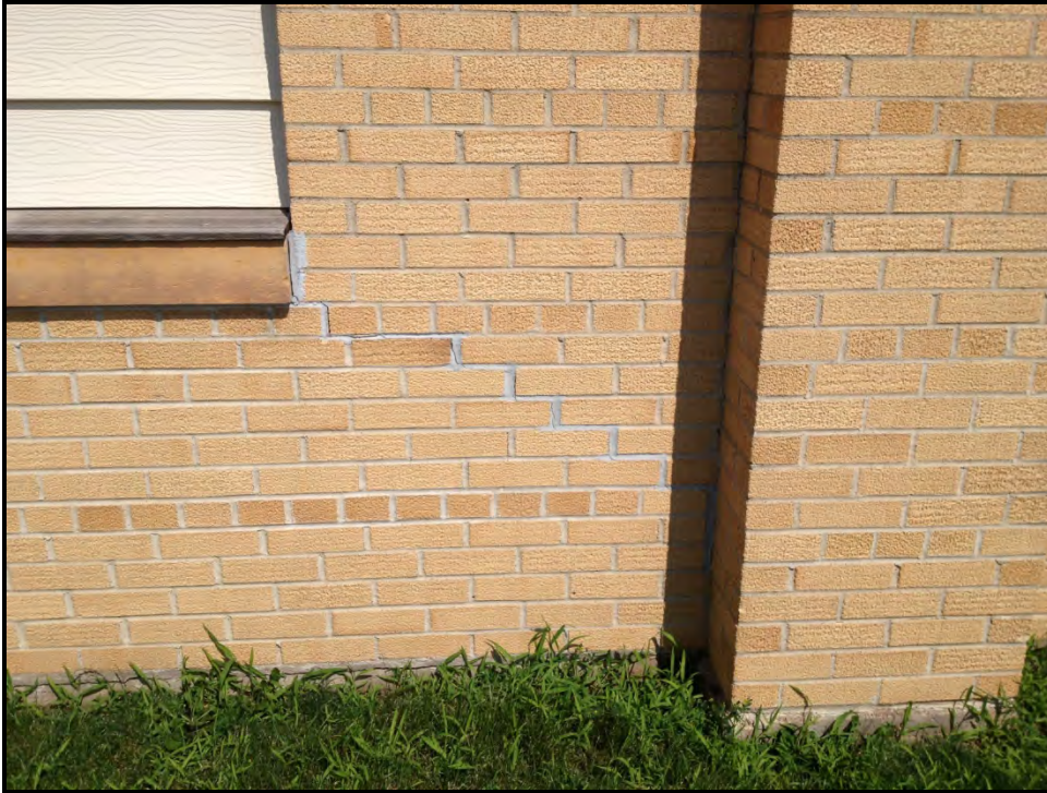
Photo #21: West Elevation – stress crack in brick veneer.
