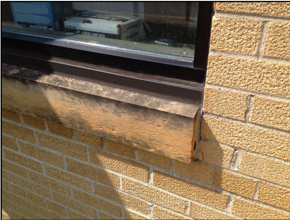
Photo #18: South Elevation – window sill condition.
