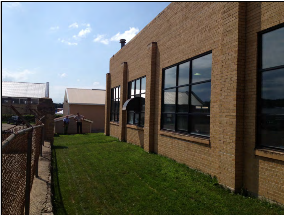
Photo #14: South Elevation – brick veneer and window sill condition.
