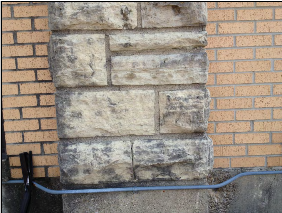
Photo #6: North and South Elevations – limestone pilaster condition.
