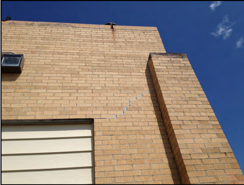
Photo #19: West Elevation – stress crack in brick veneer.
