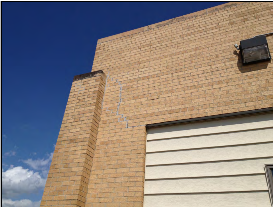
Photo #22: West Elevation – stress crack in brick veneer.
