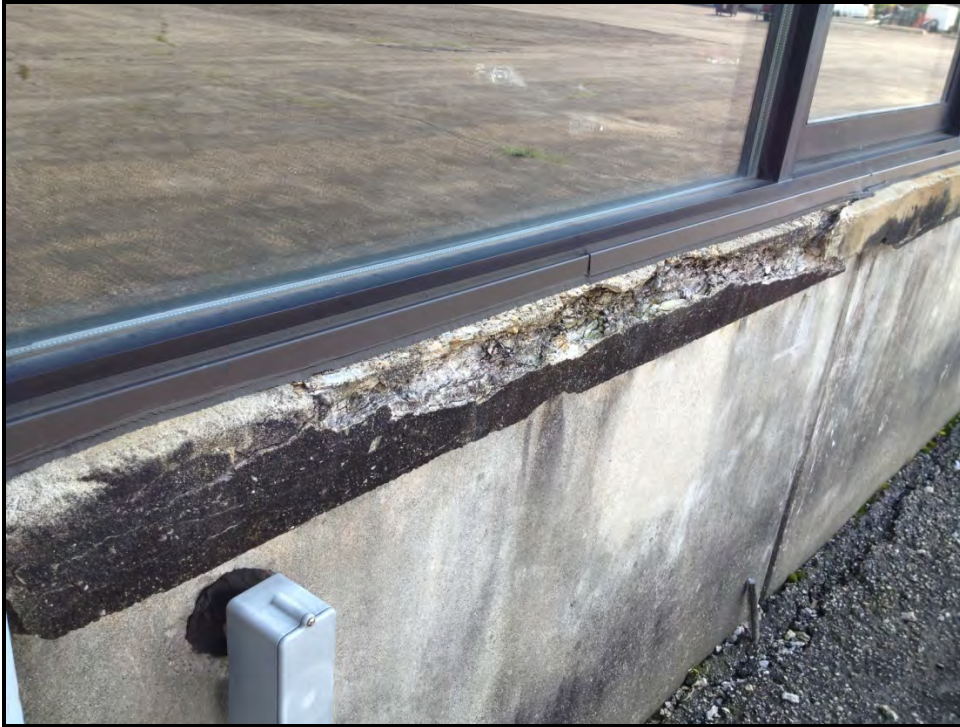
Photo #5: North and South Elevations – sill condition.
