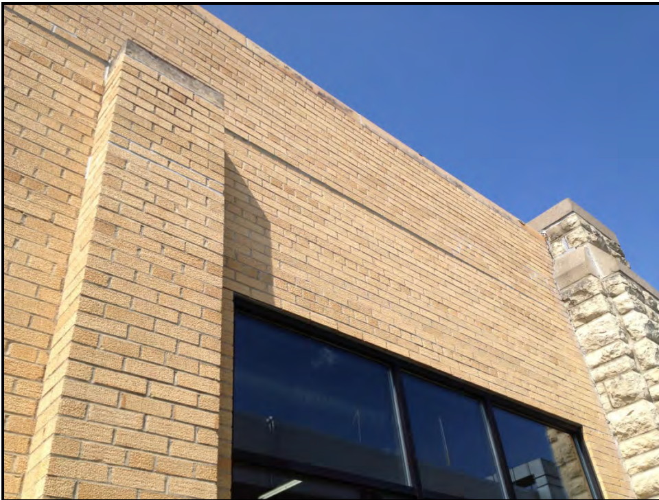
Photo #16: South Elevation – brick veneer condition.
