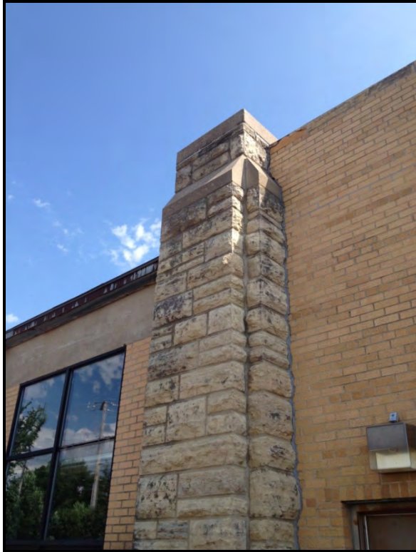
Photo #7: North and South Elevations – limestone pilaster condition.
