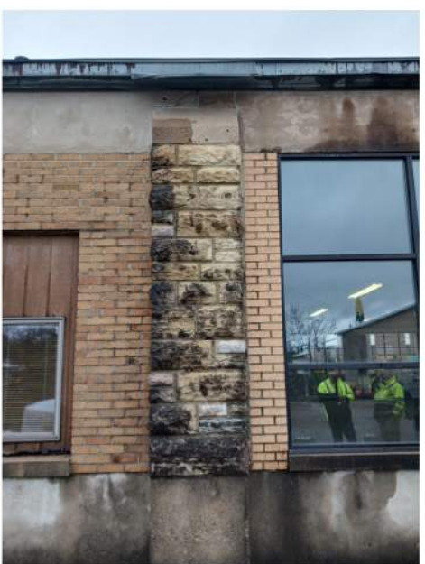
9 A201 DETERIORATED STONE NOT TO SCALE
