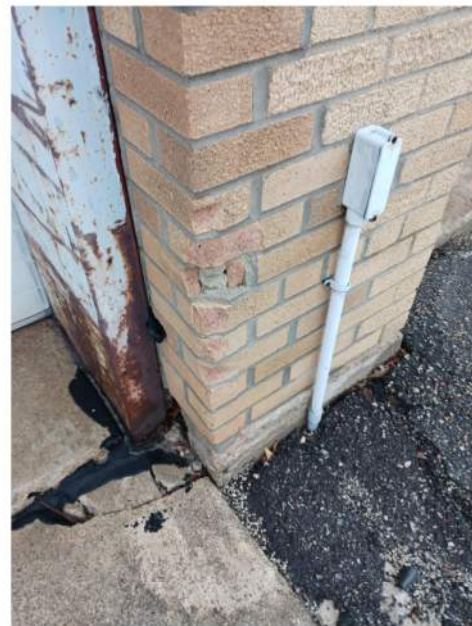
7 A201 DAMAGED BRICK NOT TO SCALE
