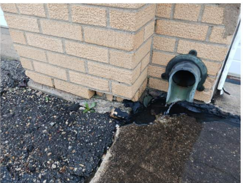
8 A201 DAMAGED BRICK NOT TO SCALE
