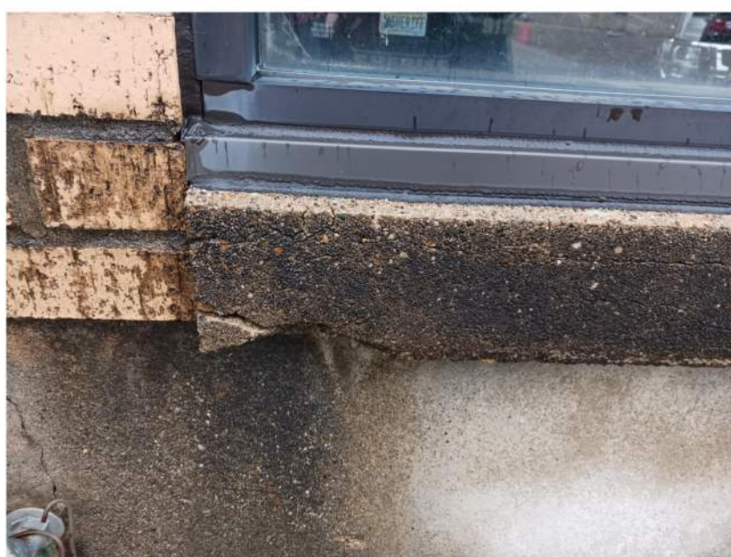
3 A201 DAMAGED WINDOW SILL NOT TO SCALE
