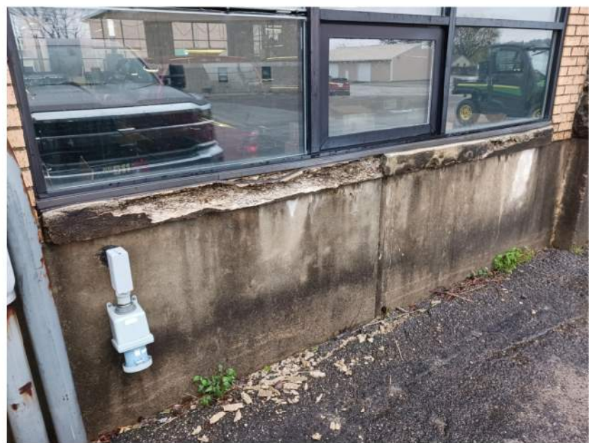
1 A201 DAMAGED WINDOW SILL NOT TO SCALE
