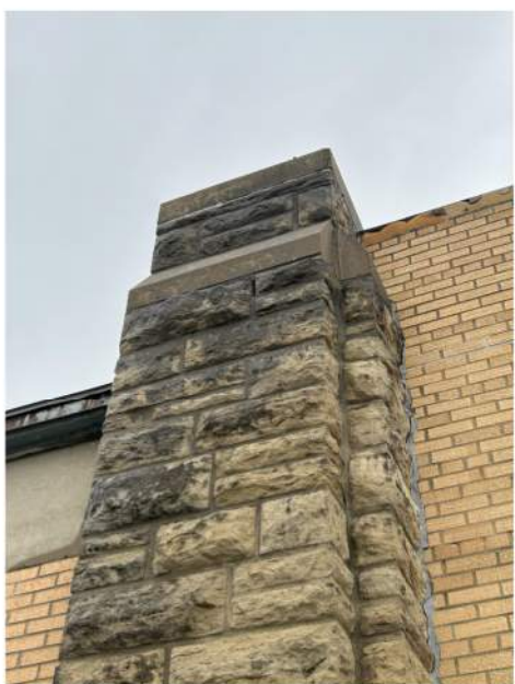
11 A201 DETERIORATED STONE NOT TO SCALE
