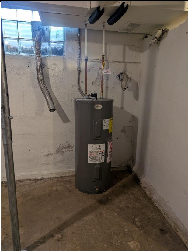
Electric water heater and clothes dryer flex duct
